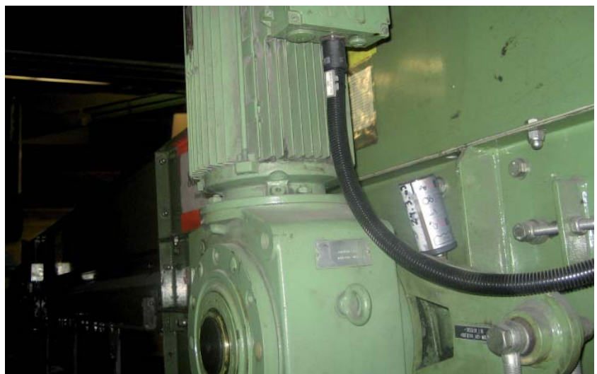
On a luggage conveyor there are many points of lubrication necessary, these are primary flanges and vertical bearings.
