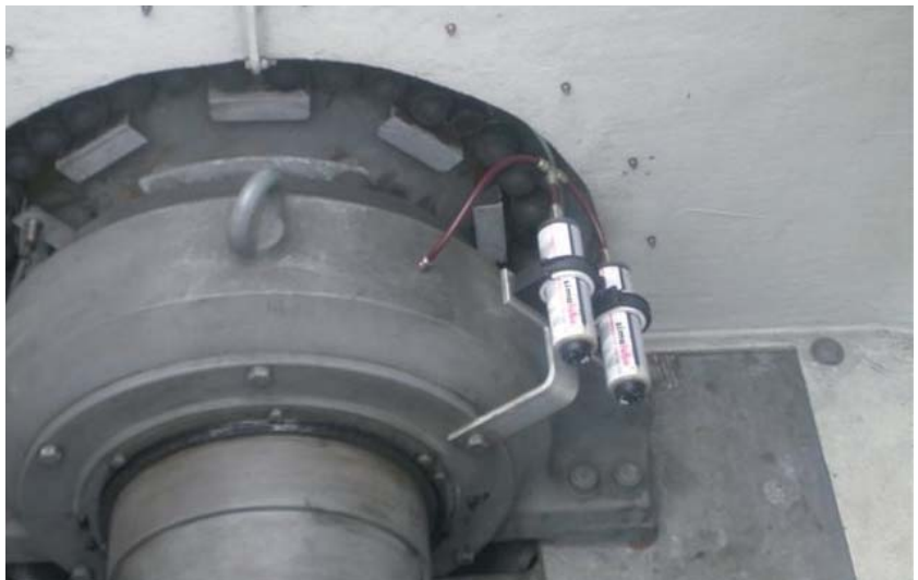
Lubrication of a primary bearing with two 250ml simalube units
